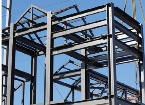
Structural Steel 2022 POY Class I Steel Fab Enterprises Amtrak Middletown, Middletown, Pennsylvania
